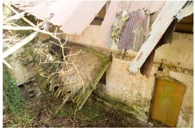
February 2010 – Collapsed Roof Structure
