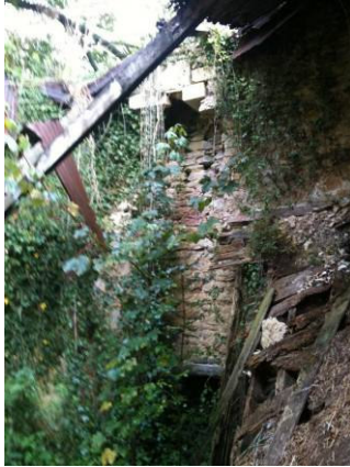
Collapsed Roof and Floor
