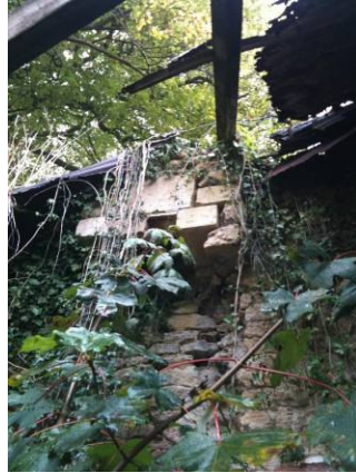
Collapsed Chimney Brest
