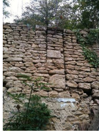
Vegetation Growth/Open Jointing
