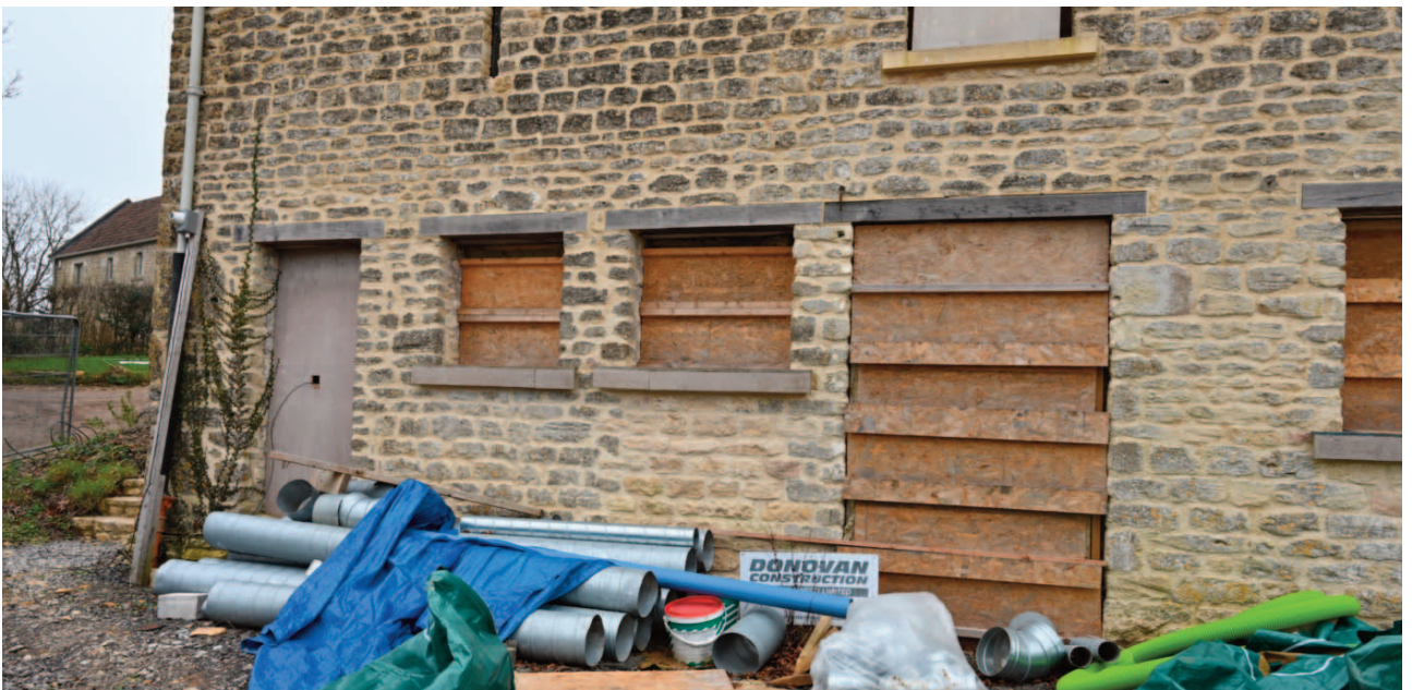
Fig. 17. The right hand window just visible here has been retained rather than replaced by a second door as approved.
