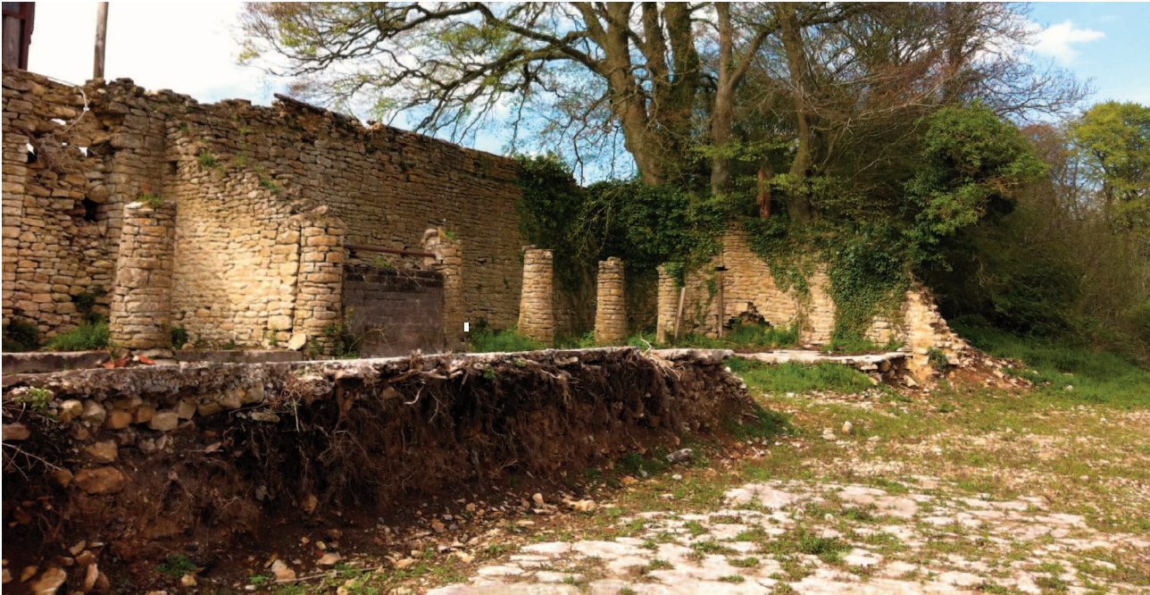
Fig 13. The former open fronted building in 2008 showing its derelict condition prior to rebuilding.
