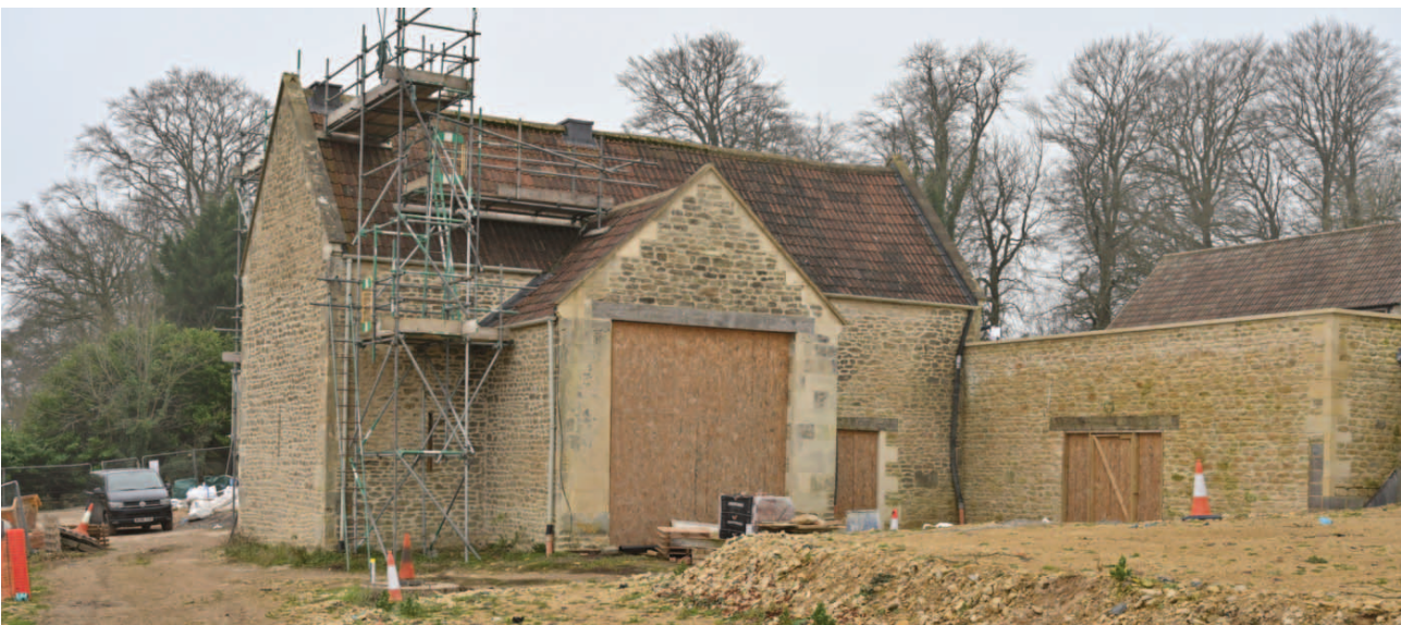
Fig. 12. The full height northeast cross barn with its off-centre midstorey and on the right the rebuilt retaining wall to the upper farmyard. The levelled material in the foreground is to be removed.
