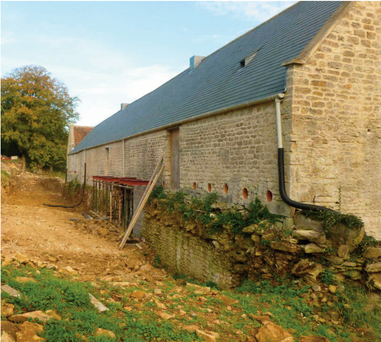
Fig. 22. The northwest wall of the barn following excavation for the 2m wide service trench and new retaining wall approved in 2016. This revealed that the southwest end of the wall was also seriously defective (as can be seen in this photograph) and this section was also rebuilt in faced blockwork to match the rest of this wall.
