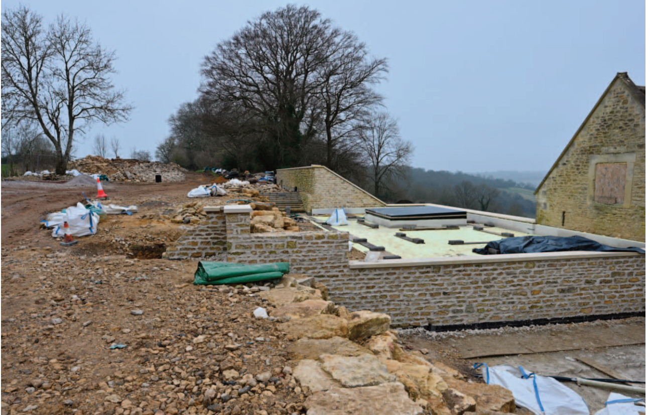
Fig. 16. The previously approved flat roofed rear extension with two rooflights rather than one, and omission of the parapet wall between the barn and outbuilding. It is proposed to install a low glass screen for safety in order to reduce the impact of the wall on the barn and former piggery range.
