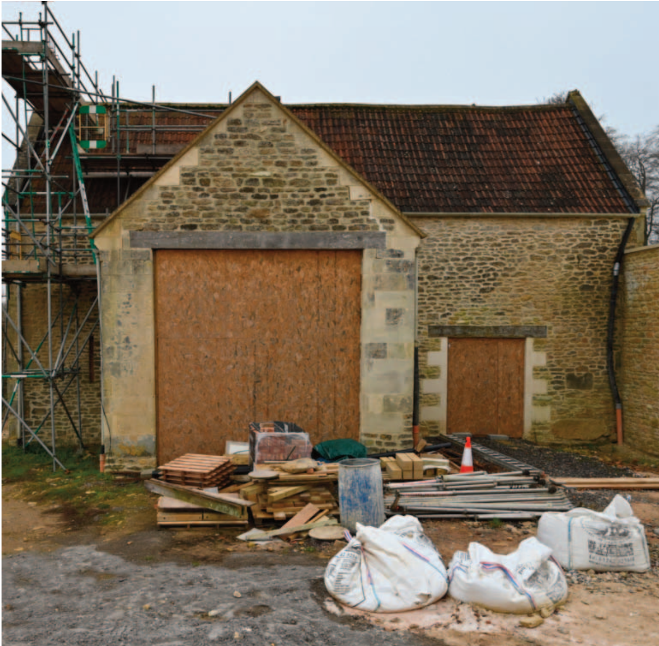
Fig. 18. The northeast elevation of the barn with the inserted opening replacing a former ventilation slot.
