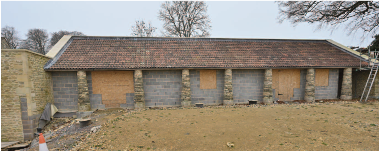
Fig. 20. The rebuilt former pig sty with its fully tiled roof and altered front wall. The omission of the glazed roof is regarded as a significant enhancement and if the render and fenestration is finished in recessive colours these alterations are considered to have an overall neutral impact on the character of the restored building.
