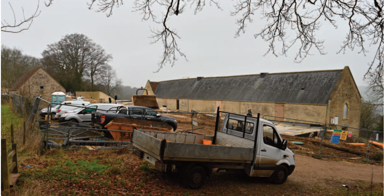
Fig. 15. The northwest elevation of the barn omitting the three approved rooflights. The electricity supply boxes on the west gable are temporary
