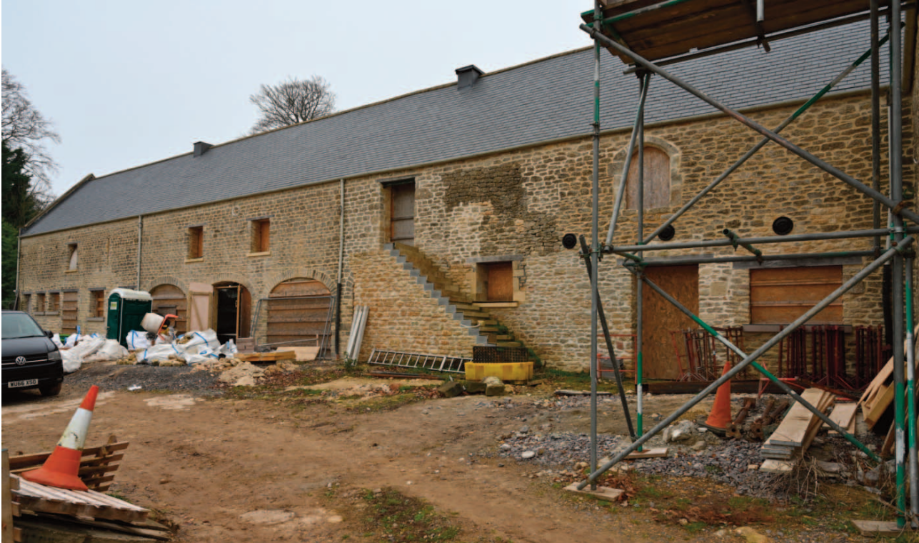
Fig. 11. The southeast elevation of the main barn, comprising the older central section with its reused arched first floor opening, and to the left of the taller steps an extension with four arched ground floor openings and a further extension to the left. The attached full height cross barn is just out of sight on the right.
