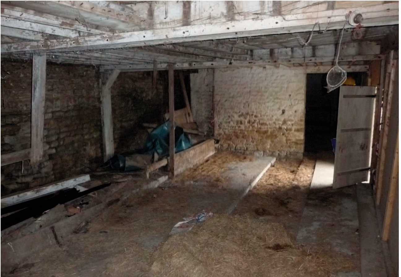
Fig. 23. The proposed dining room prior to commencement of the works with the rear retaining wall apparently in reasonable condition on the left. The first floor structure was in poor condition and approved for replacement in 2012.
