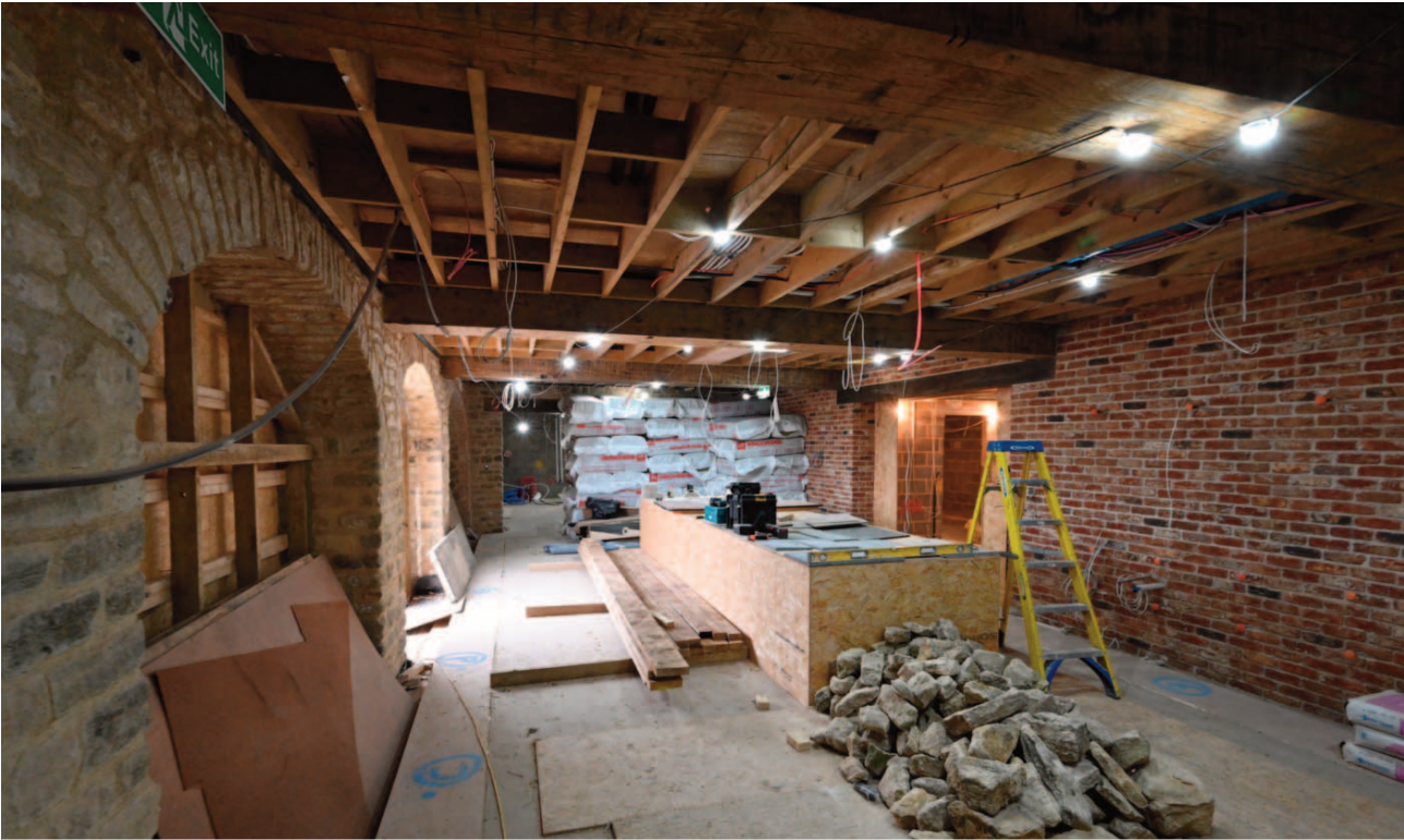
Fig. 24. The additional length of rebuilt ground floor rear wall in the new kitchen showing the new opening into the rear basement extension.. The extension walls and this section of rear rebuilt wall is faced in brick-work over blockwork.
