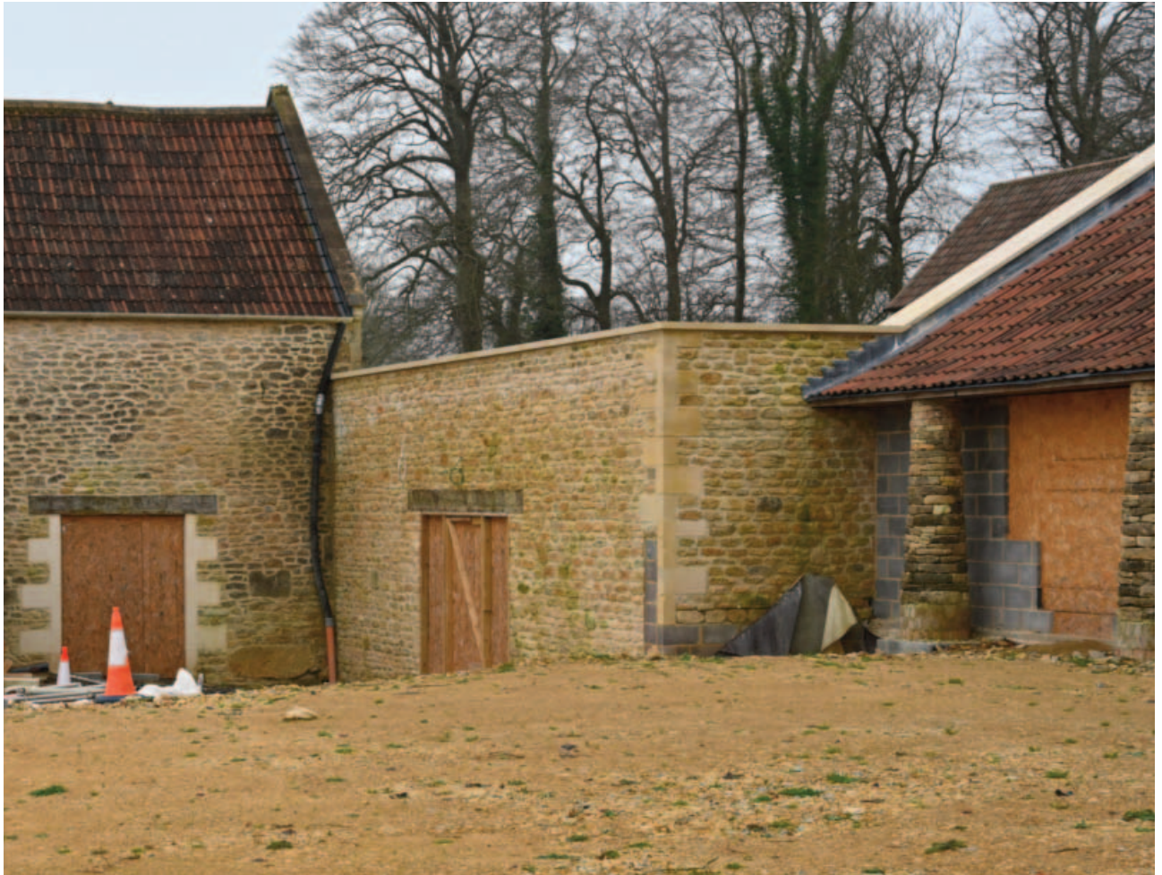
Fig. 19. The rebuilt front wall to the flat roofed extension between the main barn and the former pigsty building. The angle has been changed slightly and the wall is to have non-reflective glass parapet
