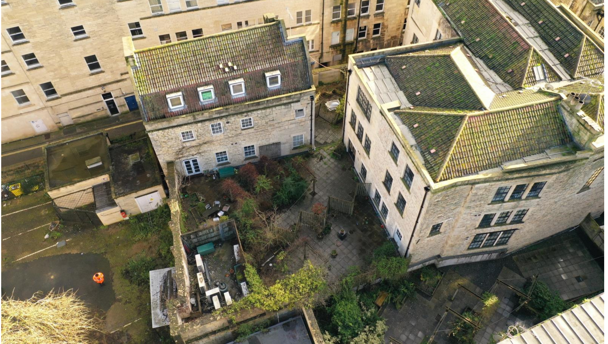
Photo 5: oblique aerial photo showing Nos. 1 and 3 Parsonage Lane in the foreground, with its enclosed courtyard garden. The north west corner of the courtyard includes a compound of condenser units servicing the retail floor space below.
