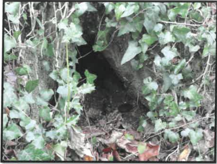
PLATE 1 - CAVITY AT BASE OF T2
