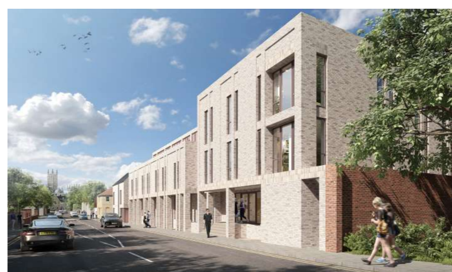
Alma Court, Canterbury 197 student rooms Associated facilities, amenity space, parking; access and areas of landscaping. Currently in build, due to be completed in 2020
