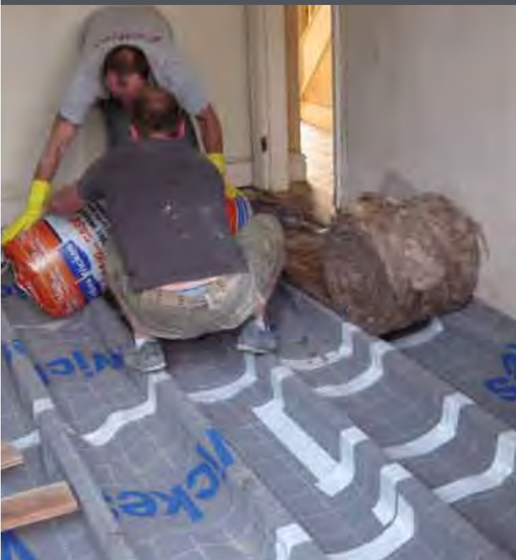
Insulating a suspended timber floor from above: the breather membrane provides excellent draught-proofing as well as support for the insulation
