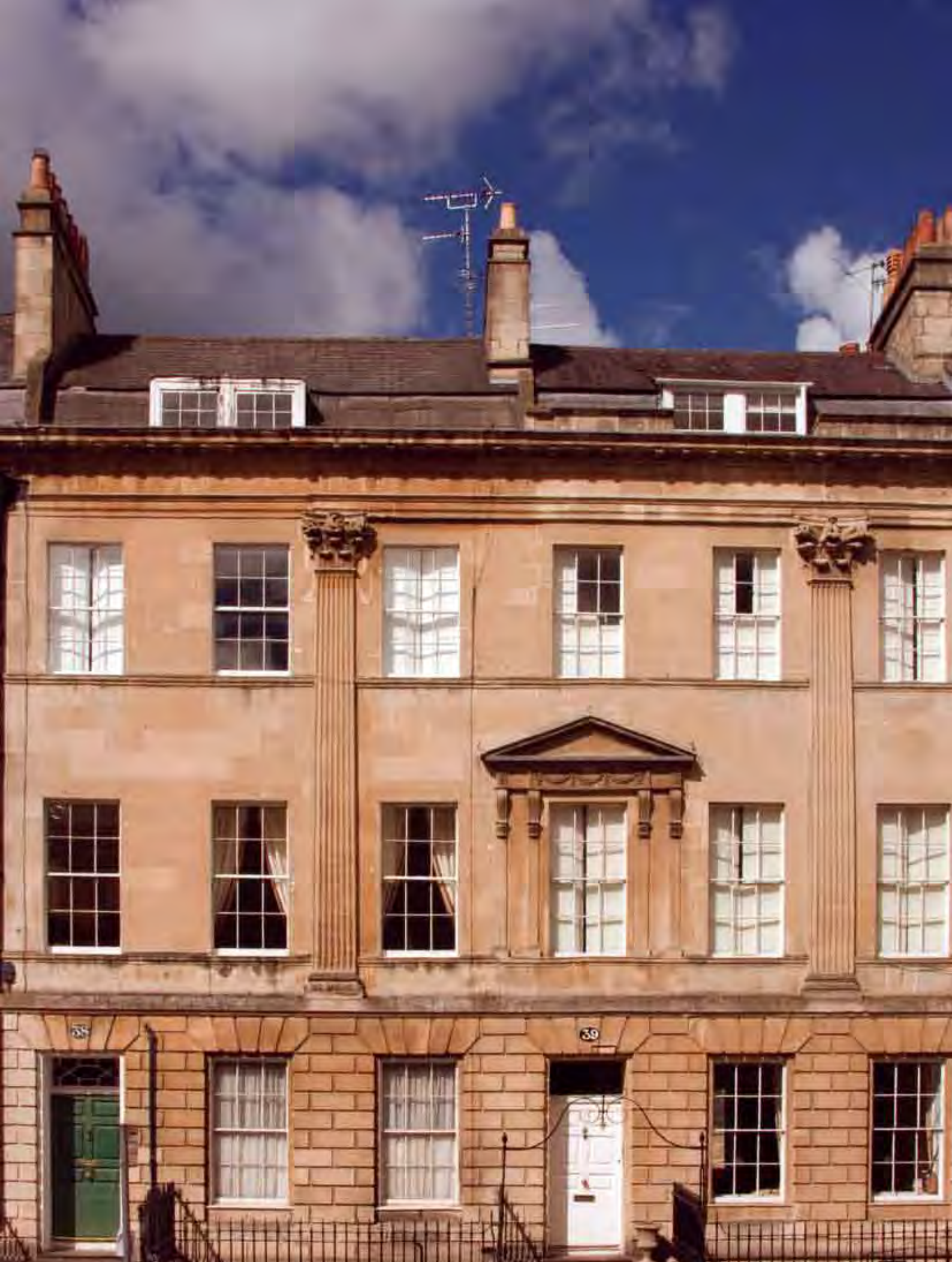
The heat loss through these elegant sash windows in Great Pulteney Street is reduced by the use of shutters and curtains (but only when they are closed)
