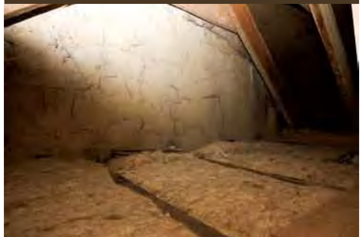
Sheep's wool insulation laid between the joists of a loft space in a late Georgian house on Bathwick Hill
