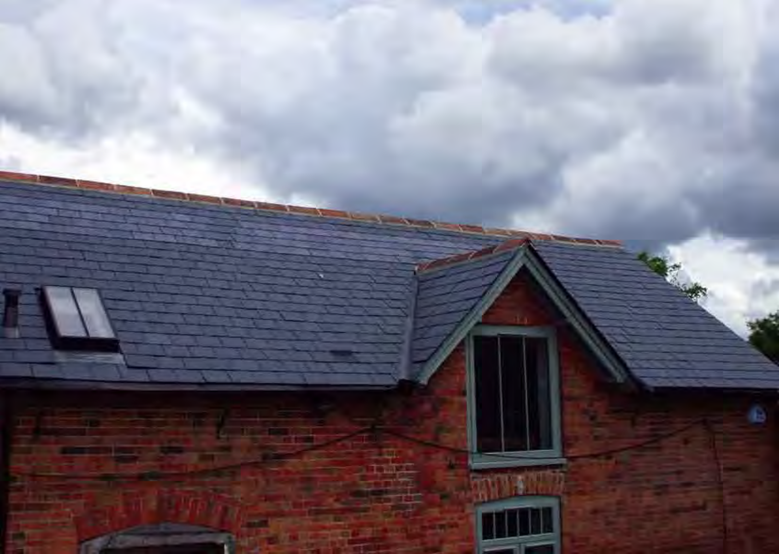
Photovoltaic 'solar slates' can just be distinguished from the real tiles on the upper part of the roof of this Grade II listed farmhouse in Wiltshire
