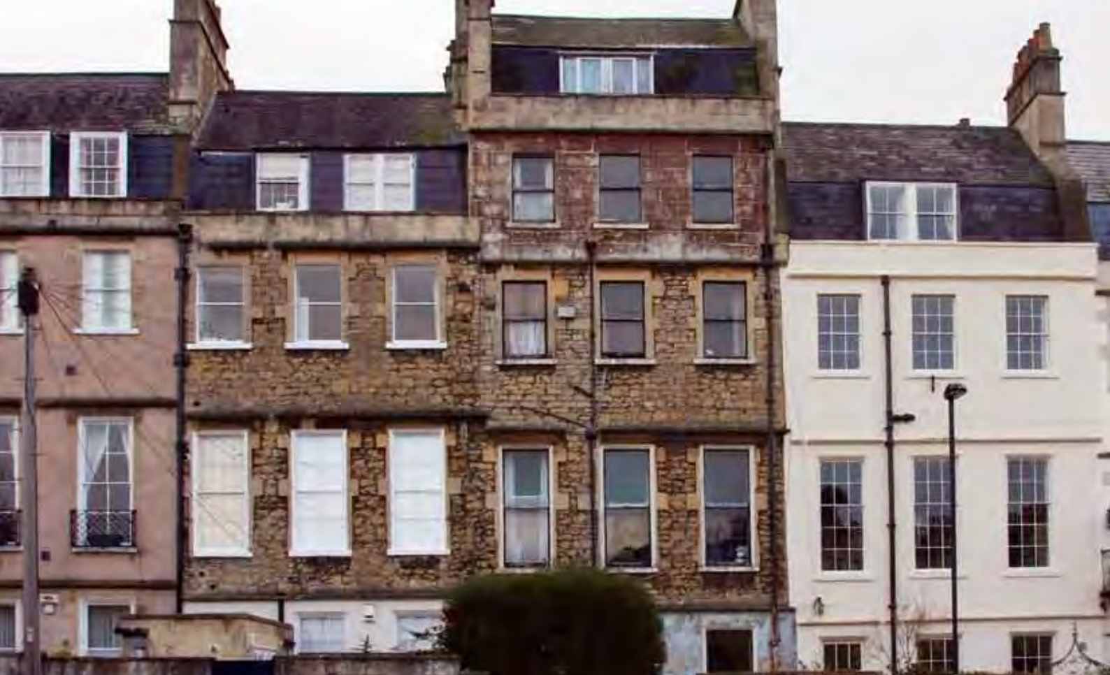
Many of the rubble-stone rear facades of the Georgian houses of Bath were originally rendered. External insulation could be used in such instances to return the facades to something closer to their original appearance.
